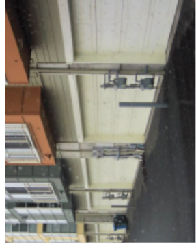
Exposed utility meters like this will not be allowed where visible from common open spaces, streets or pedestrian areas.
