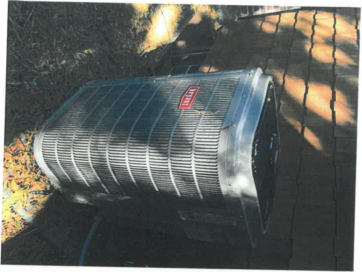
Air Handler and Heat Pump
