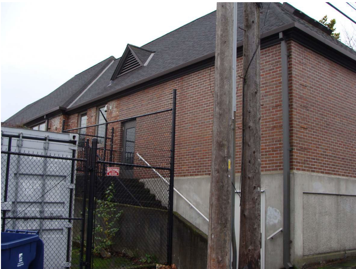
Figure 18. Northwest (rear) corner of the north wing of the Mottet Library (McClintock, 2021)
