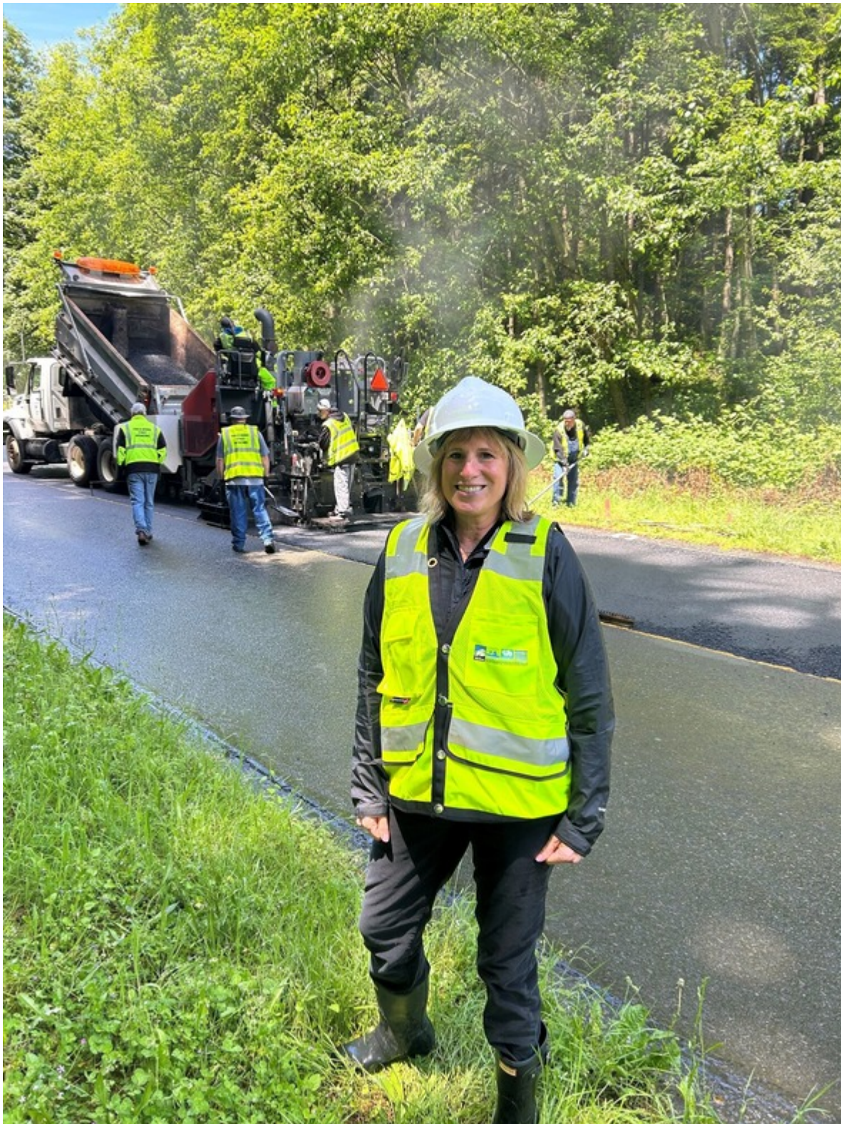
I joined our Tacoma Public Works Department as they worked to replace and fill parts of Northshore Parkway in NE Tacoma.
