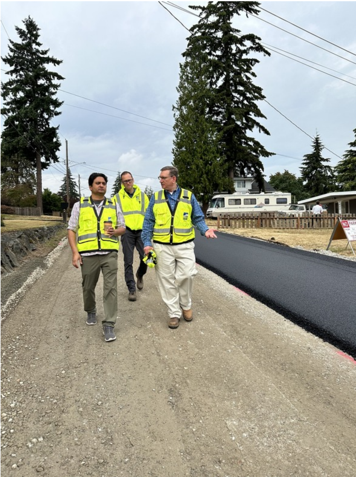
One of the main responsibilities the City has is to maintain our roads. I joined our public works staff on E 45th and E I Street to watch a repaving project.
