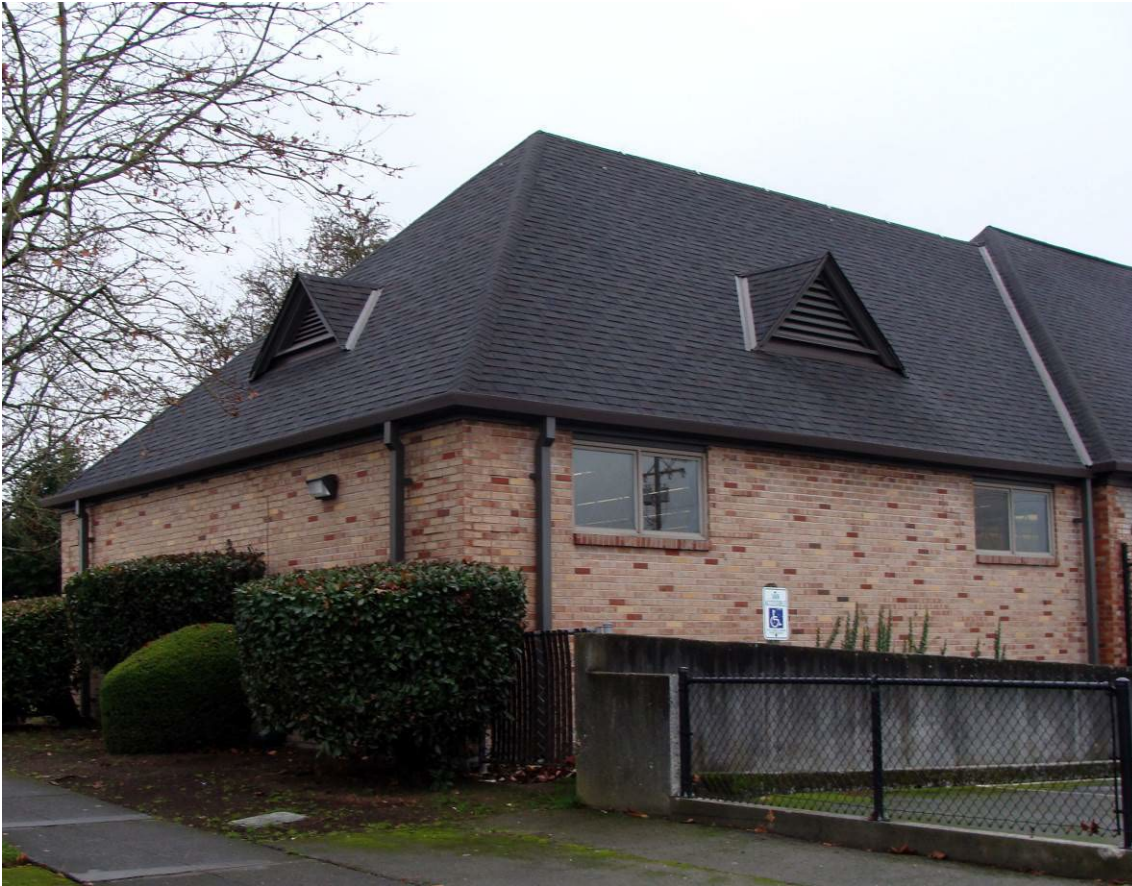
Figure 15. Northeast rear corner of the south wing of the Mottet Library. (McClintock, 2021)
