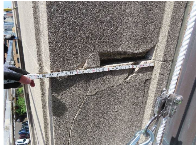
Cast Stone Condition Credit: WJE Associates, Inc.
