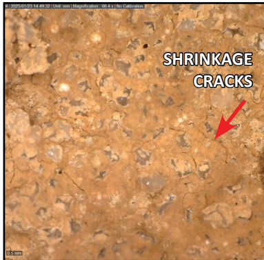
B1 - CATHEDRAL STONE Aggregate very difficult to see through mortar cream. Shrinkage cracks throughout.
