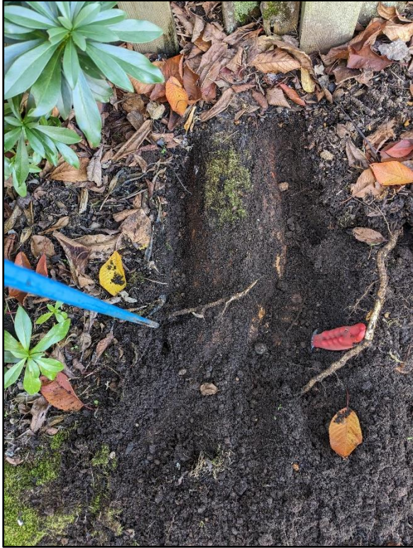
Photo 2: Structural root extending from base of Tree 1 east toward proposed sewer line/948 house.
