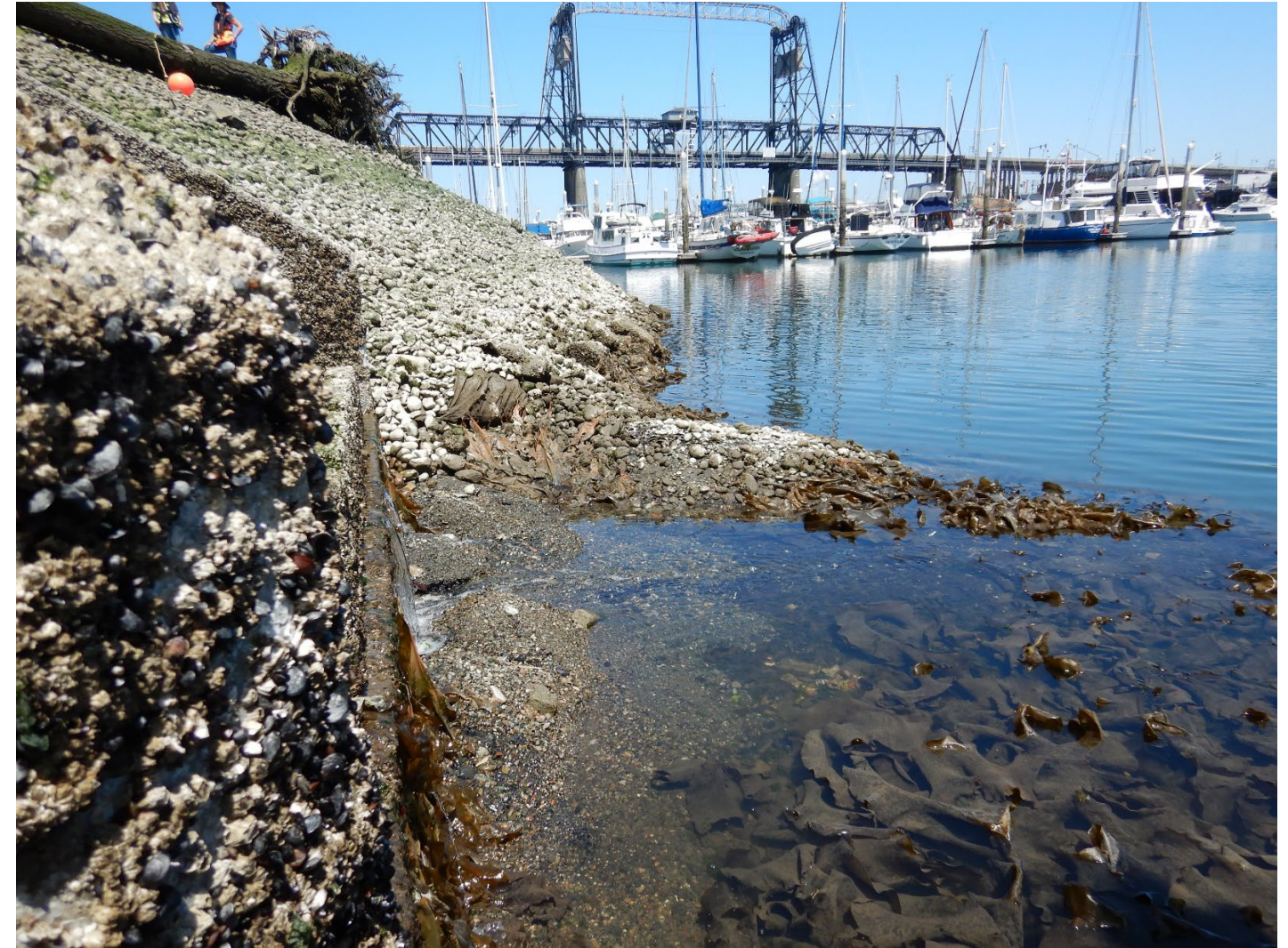
Photograph 2. City Outfall 230A apron along the Thea Foss and Wheeler-Osgood waterways west bank during the Year 17 low-tide slope cap inspection as part of the Long-Term Monitoring Plan (LTMP) taken at -3.1 feet MLLW. Loss of slope cap material, round river cobbles, placed off the outfall apron exposing geotextile, gravel, and sand below top ledge of the apron.
