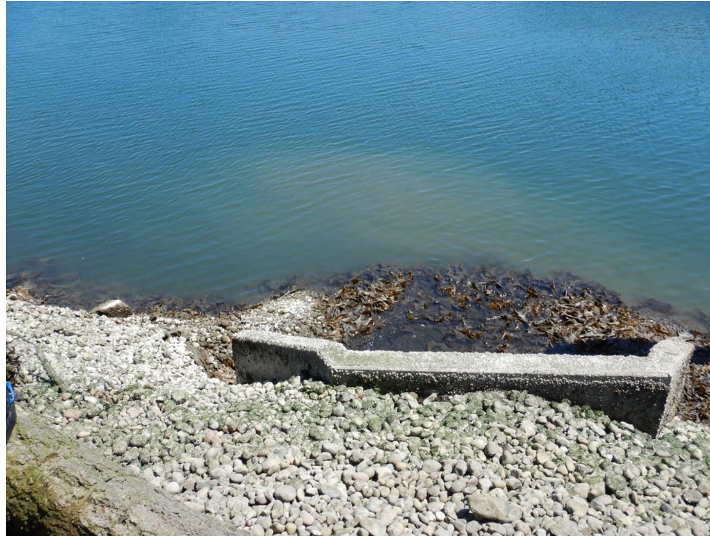
Photograph 3. City Outfall 230A outlet structure from farther up the slope taken during the Year 17 slope cap inspection as part of the Long-Term Monitoring Plan for the Thea Foss and Wheeler-Osgood waterways taken at -3.1 feet MLLW. Loss of slope cap material, round river cobbles, placed off the outfall apron exposing gravel and sand below top ledge of the apron.
