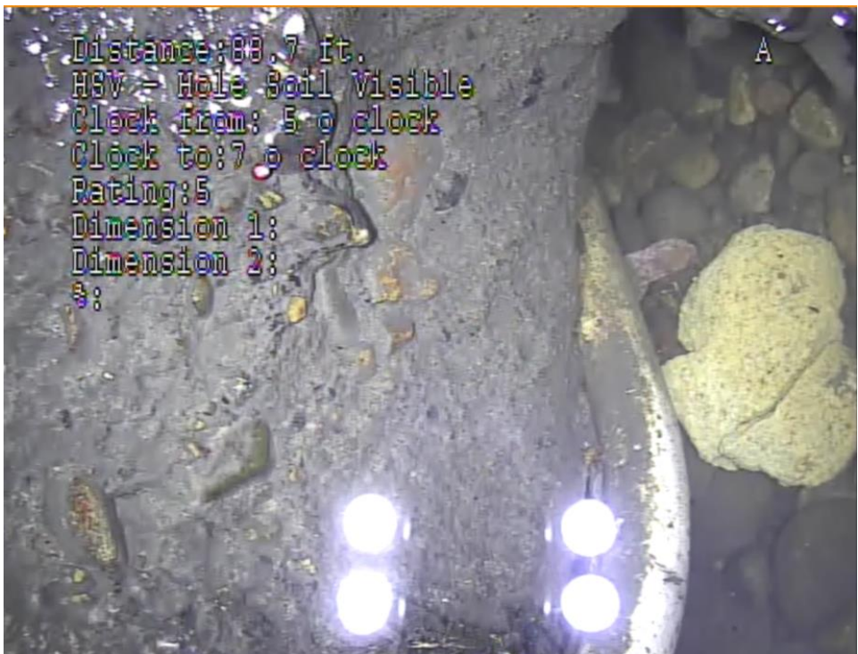
Spot Repair liner at 88.7 LF Upstream to 92 LF Upstream in front of 1002 S 38 th St (7-11 Store)
