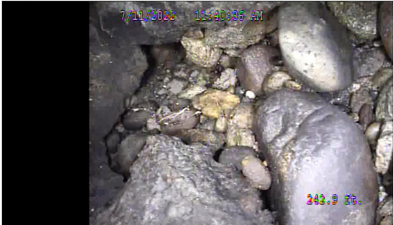
Close up view of the hole in the side wall at 242.9 LF Downstream at Spot Repair Lining – joint to joint
