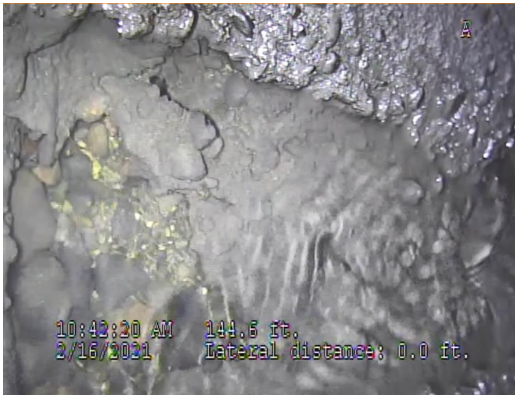
Spot Repair liner at 144.6 LF Upstream to 147.6 LF Upstream in front of 7-11 store
