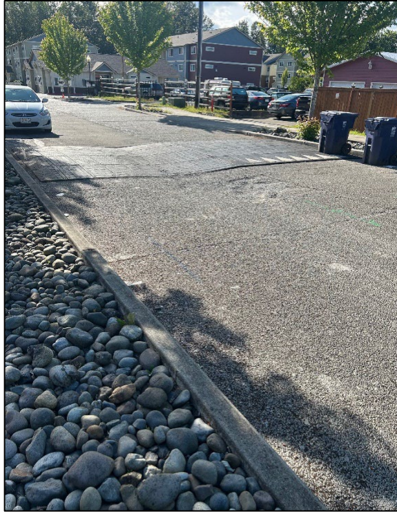
Photograph 1. Settlement and distressing in southern half of South 38 th Street, looking northwest.
