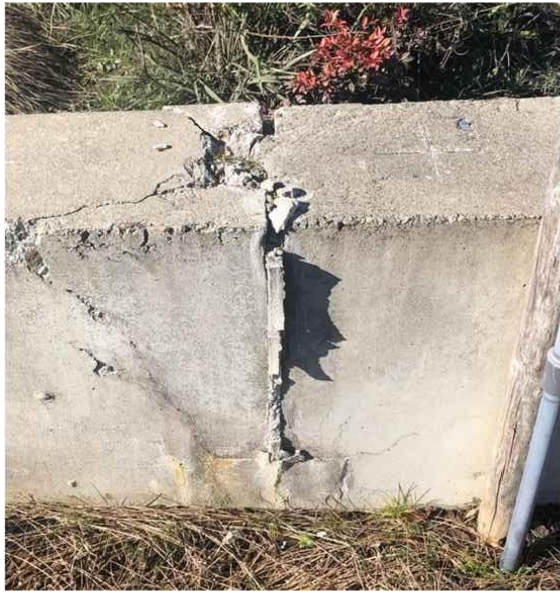
Figure 2: Typical Joint Spall
