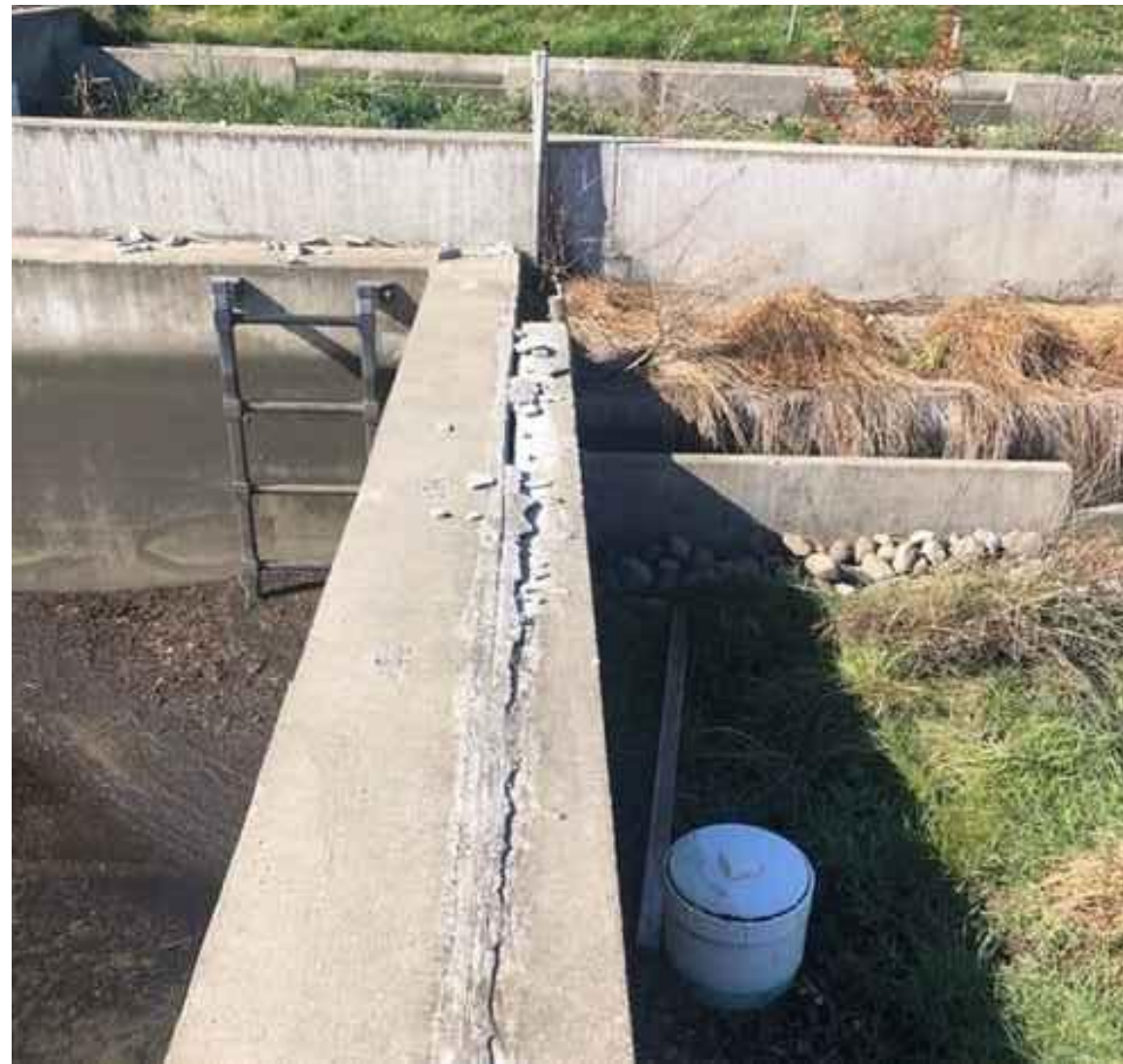
Figure 6: Typical Horizontal Joint Failure
