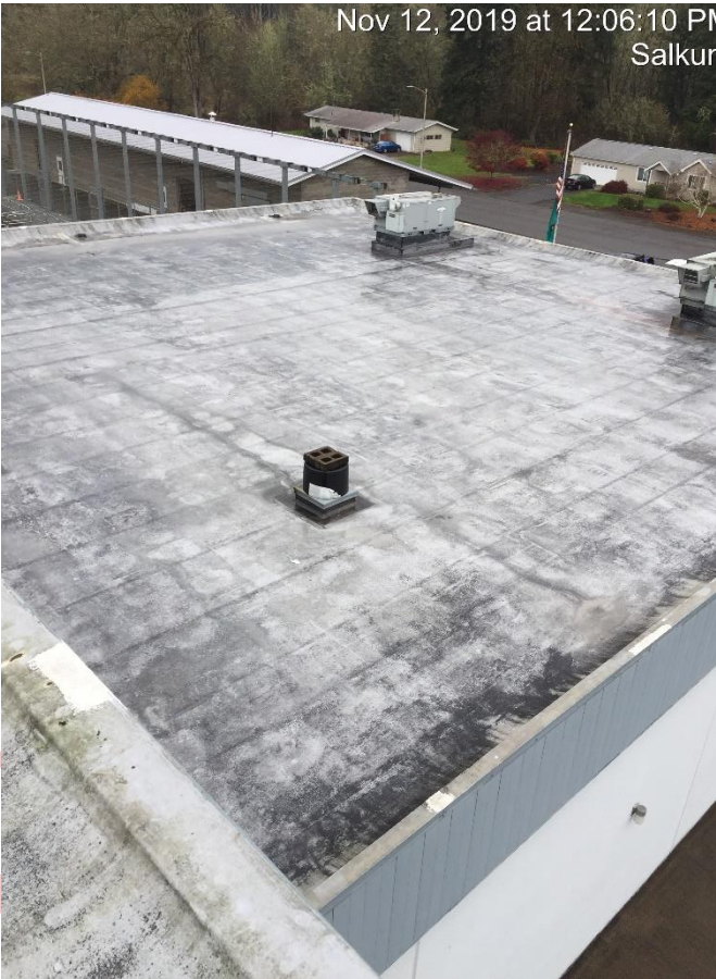
Kemper System-1 piece membrane roof over-coat system (easterly roof)
