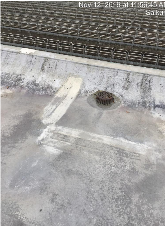
Old misc repairs
