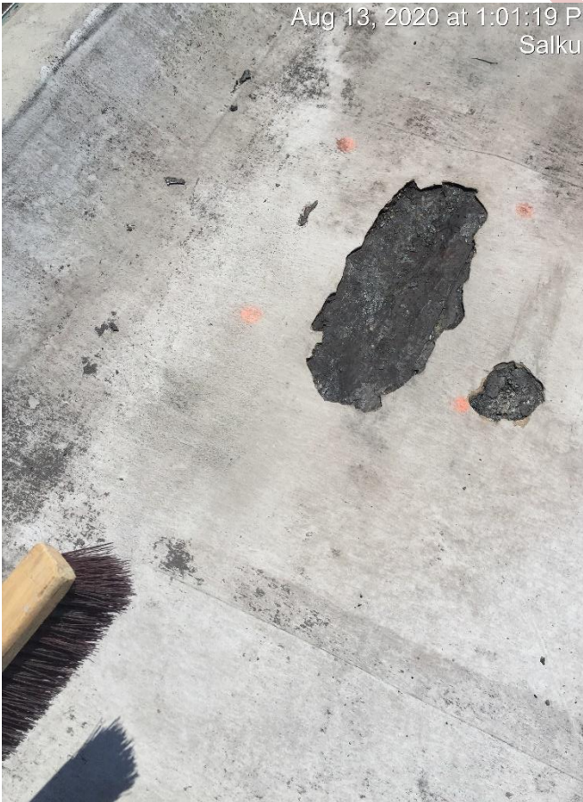
Silicone and Kemper System over-coatings removed exposing the old liquid-asphalt roof coating
