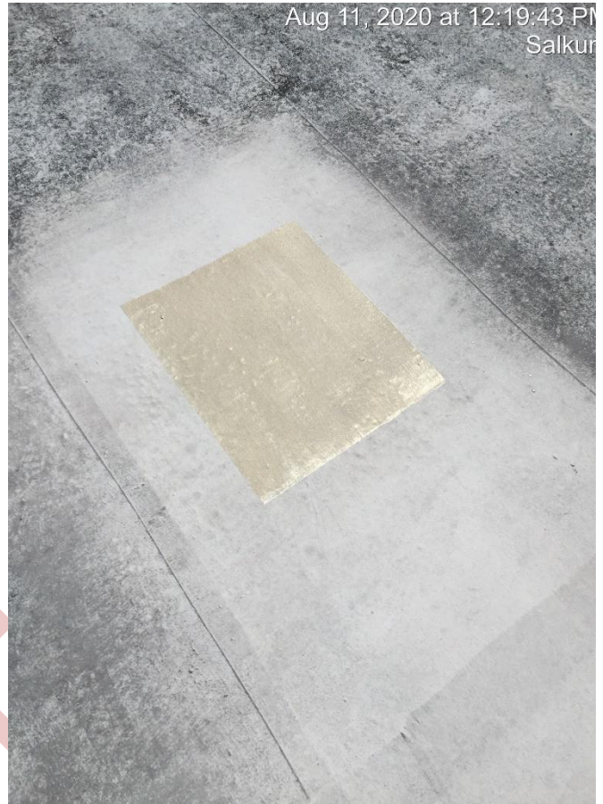
Henry's 555 Fibered Aluminum Coating applied directly over the existing silicone maintenance coating
