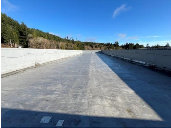
View SW of Cushman 2 Powerhouse. Upper roof to be reroofed, Annex to be reroofed and awnings upper and lower to be reroofed.
