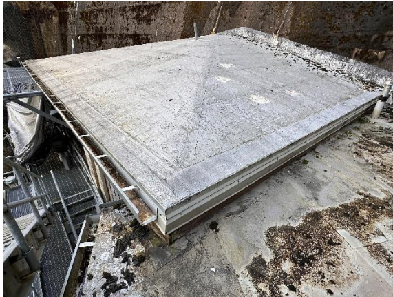
View of the roof of Valve House roof, gutter and roof material to face of dam.
