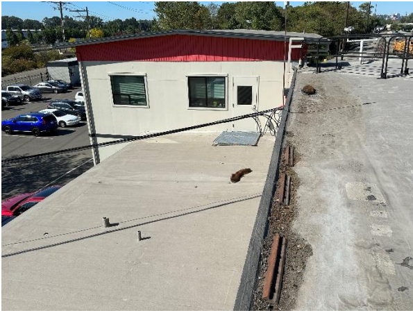
View west, roof 1 (right side), roof 3 (left side), roof 7 in the background.
