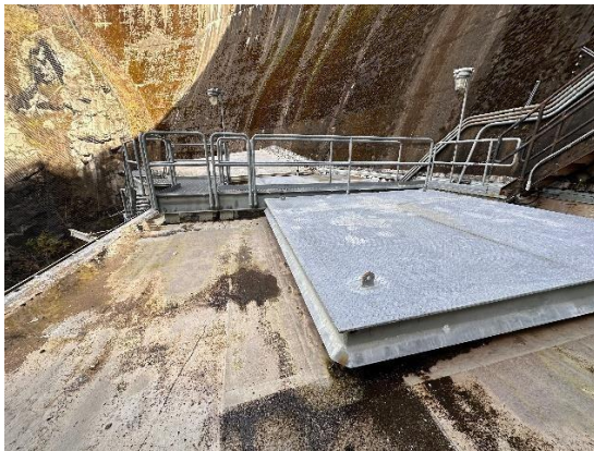
View of NF Powerhouse hatch covers, roof protrusions, walkway and connection of roofing material to the dam.
