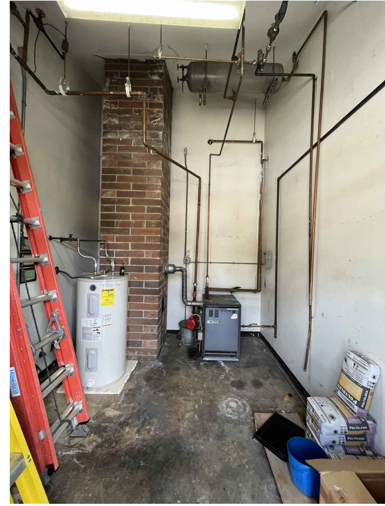
(E) HEATER ROOM
